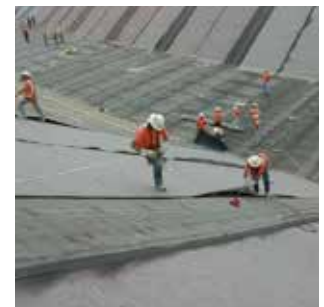
Torch welding of seams does not require special equipment or the use of chemicals for bonding.
