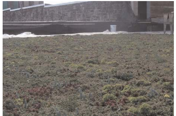
Photo 6 - Four Months After Installation
